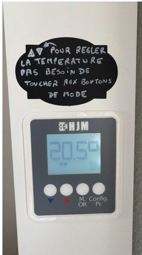
living room heating
